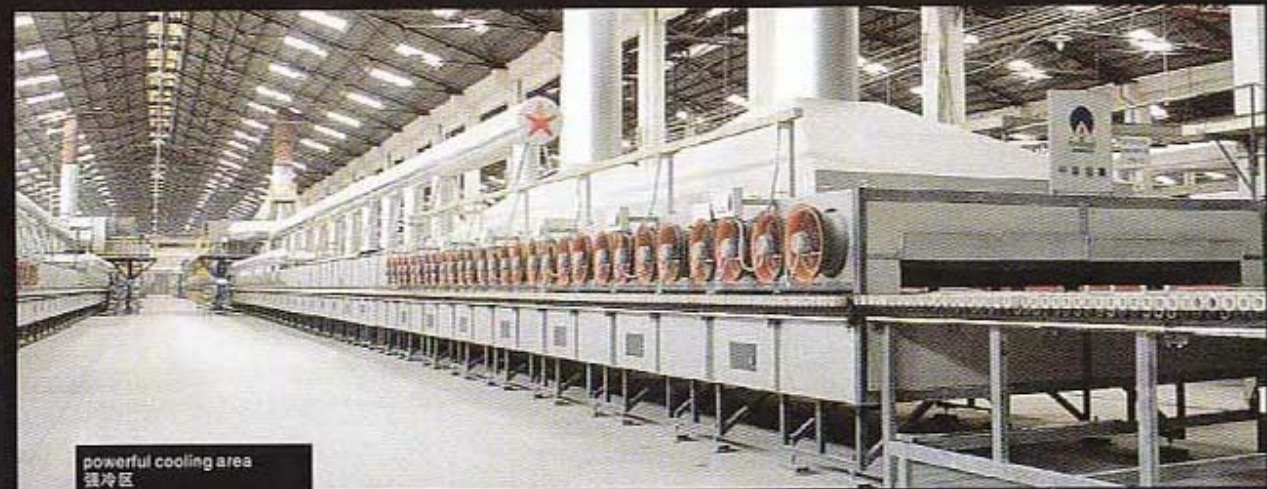
Indirect cooling area 间冷区
